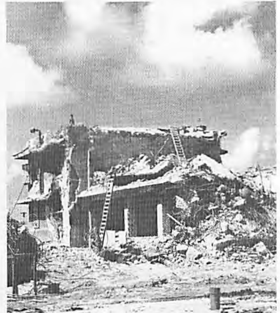
Demolished Japanese headquarters building.
